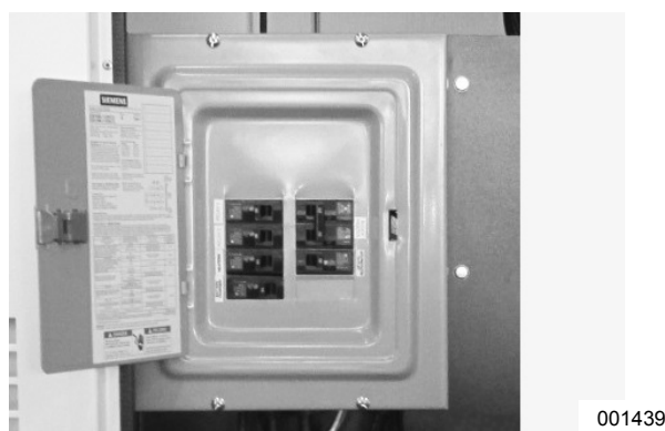
Figure 3-2. Circuit Breaker Box
